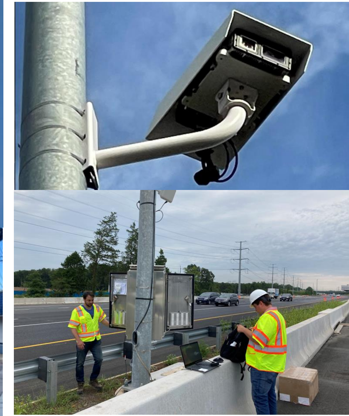
Customer B – I-66, Virginia Automated Incident Detection
